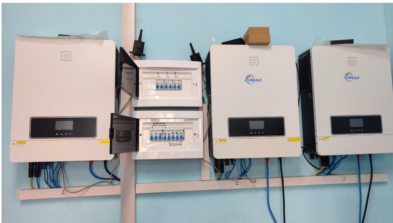
Figure 8. Connection box of the Hybrid FES installed in the 4 th general secondary school of Mingbulok district.
