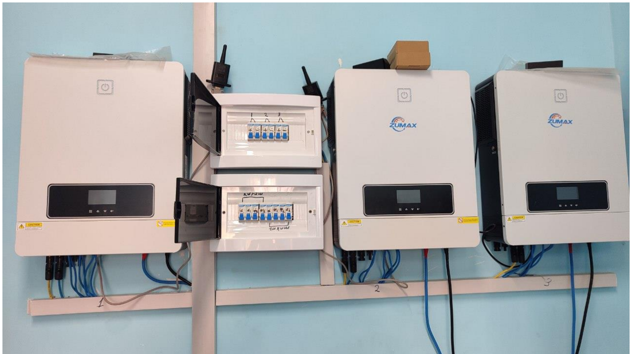
Figure 8. Connection box of the Hybrid FES installed in the 4 th general secondary school of Mingbulok district.
