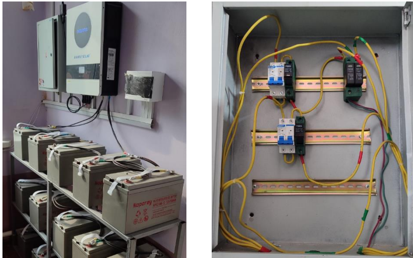
Figure 9. FES inverters and a junction box installed in the 14 th general secondary school of Mingbulok district.
